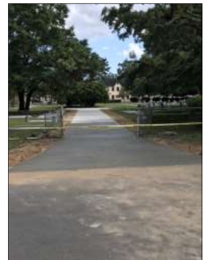
Cemetery Upgrade Completed The drive at the cemetery has been paved to ease access from Strong Street into the property.
